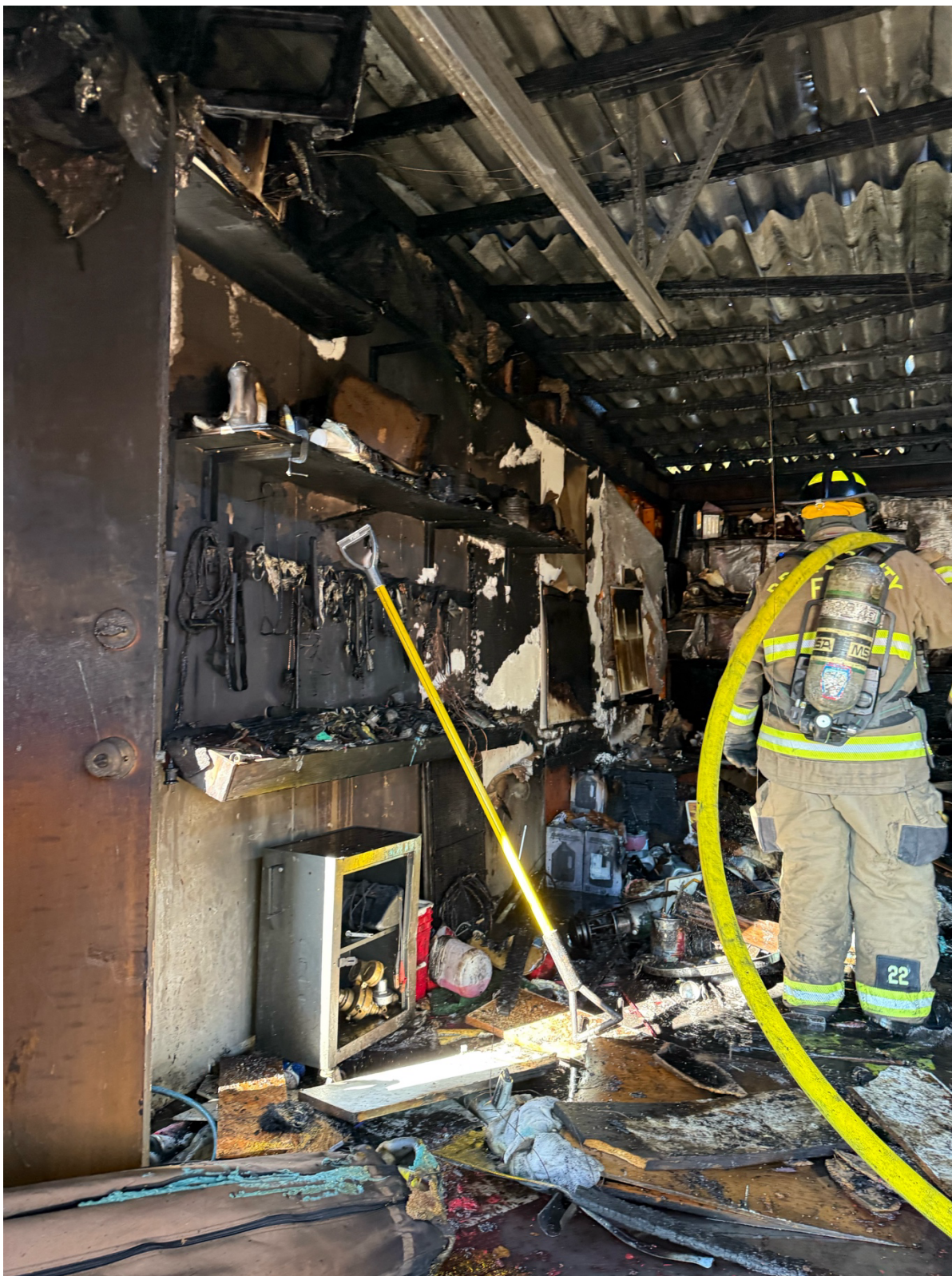
Image 2 - View of the B (bravo) side of the interior garage where the fuel was stored
