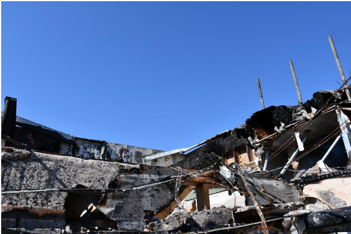
Figure # 50 Looking at a burn damage from below in 4 th floor
