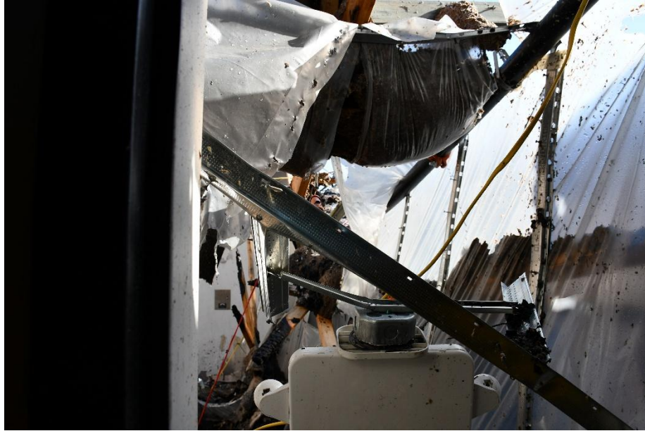
Figure #5 Looking into the 4-floor lobby elevator access area / area of collapse.
