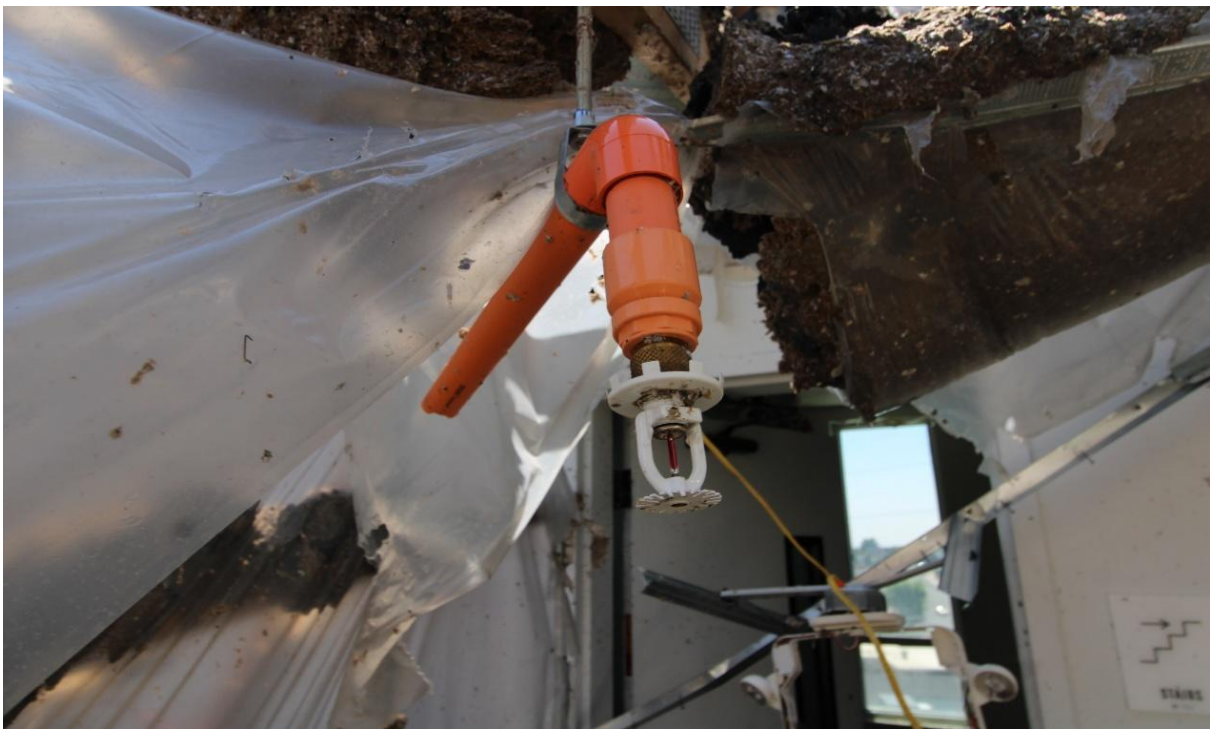
Figure #18 Looking at the Fire Sprinkler system
