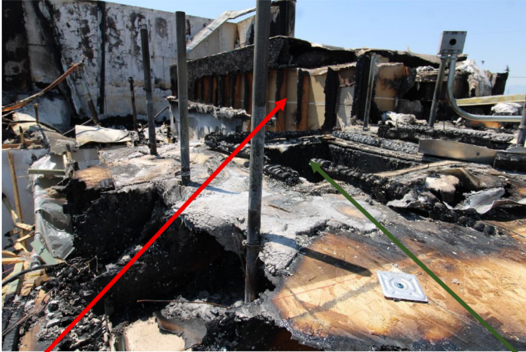
Figure#35 Looking at the burn patterns from Hallway towards the elevator
