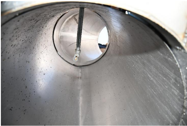
Figure 26 Looking up at the fire suppression system within
